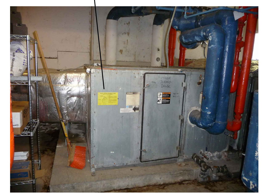
2 EXISTING OAHU-1-NW IN PENTHOUSE
